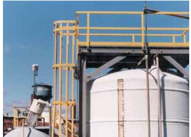
This fiberglass ladder and cage provide worker access to a maintenance platform at a Ciba Geigy plant in the northeastern United States.
