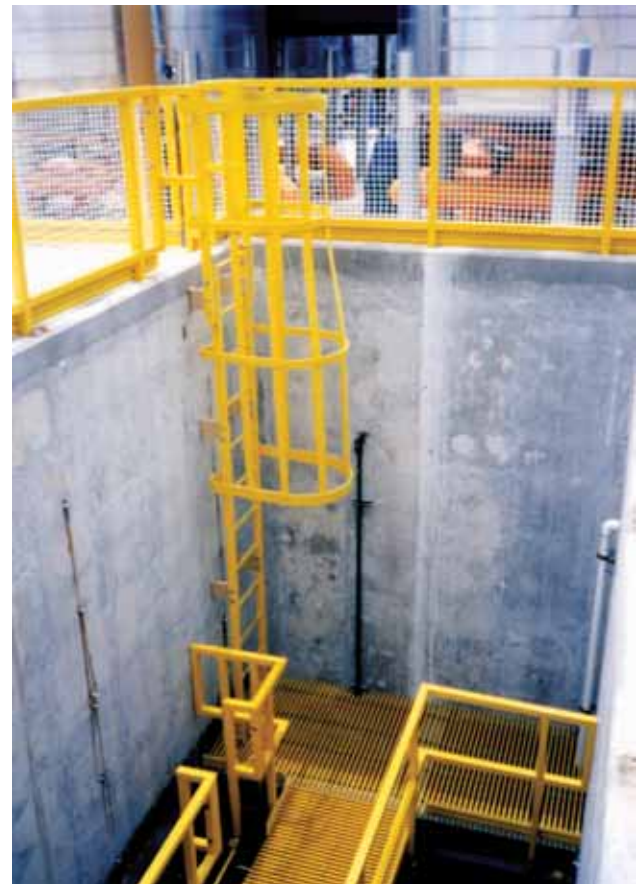
Fiberglass access ladders are used throughout the service areas of Sea World in Orlando, FL, and resist saltwater corrosion and reduce maintenance costs.
