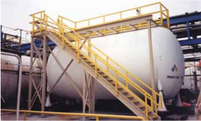
SAFRAIL™ system in a chemical plant.
