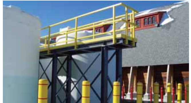
Fiberglass platforms at the Road Division of Franklin County, Ohio use SAFRIL™ square handrail around tanks that contain de-icing fluids which are extremely corrosive to metal.
