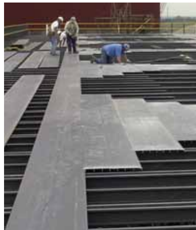
Deteriorated Plywood Fan Deck
