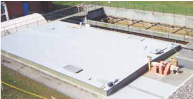
SAFPLANK® odor control covers at a wastewater treatment plant in Smithfield, RI, will withstand the corrosive environment, providing years of trouble-free service.
