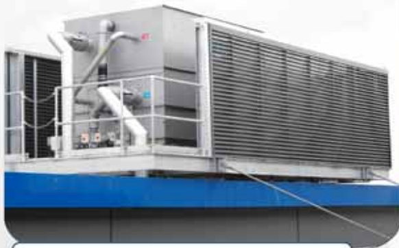
Free Cooling Chiller Unit
