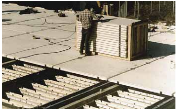
Above: A pulp plant in Canada replaced 70' x 120' corroded wooden covers over anaerobic digesters with fiberglass covers to satisfy government regulations. EXTREN® and DURASHIELD® were used to fabricate the covers. Design prefabrication and supervision of installation was completed by Strongwell.
