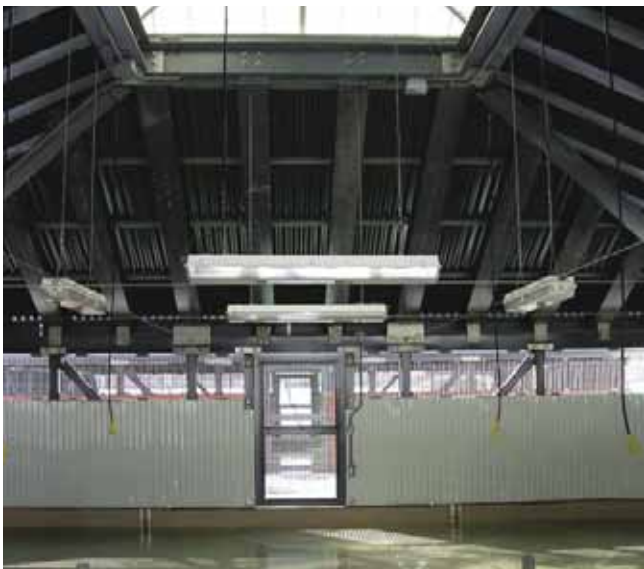
Above: The Craig Brook National Fish Hatchery in East Orland Maine used corrosive-resistant EXTREN® structural shapes to frame roofing structures over moisture rich crowding pools.
