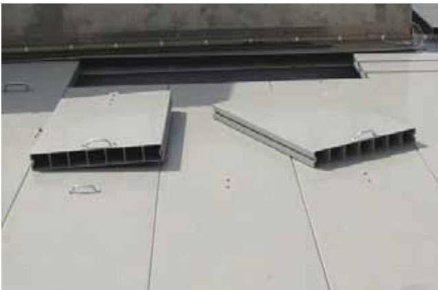
Above: A COMPOSOLITE® fiberglass building panel system functions as a clarifier cover in East Helena, Montana. The composite building panels were selected to prevent freezing during the winter and reduce algae growth in the summer months.
