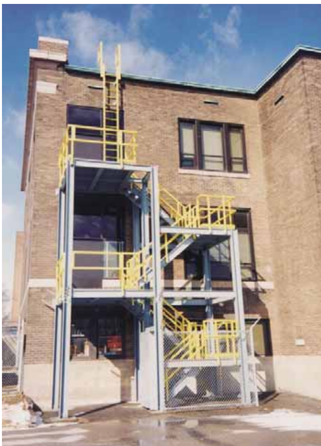
Above: FRP was chosen for this three-story fire escape because fiberglass would not require painting or maintenance.
