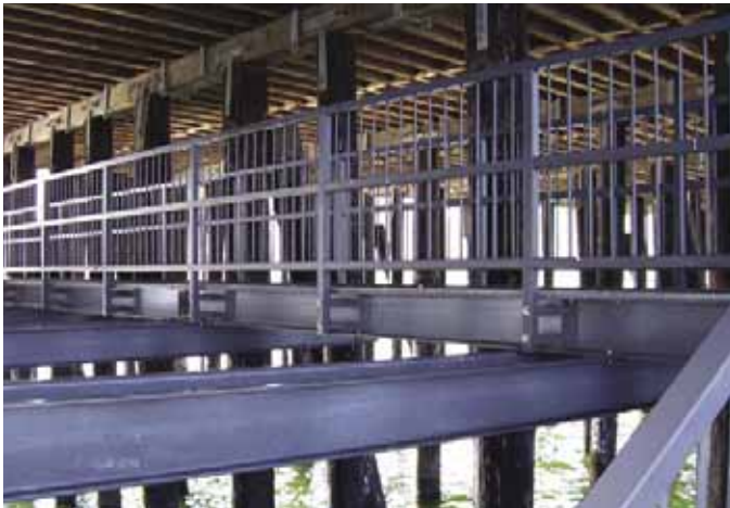
The Avila Beach Pier in California was reconstructed using EXTREN® structural shapes for support, DURADEK® pultruded grating, stair treads and custom handrail.
