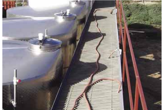
Strongwell's pultruded grating replaced rusted grating in a catwalk system for a California winery.
