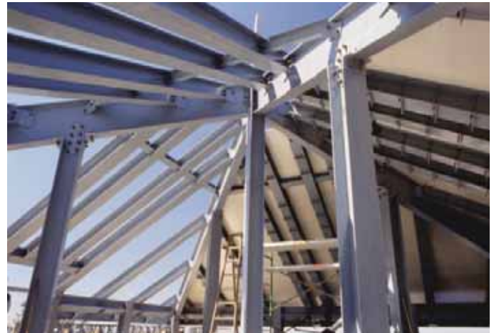
A fiberglass fabricated roof tops the Aerial Tram Station on Stone Mountain, Georgia (as seen on the cover). Concealing over 20 antenna, the fiberglass structure comprised of EXTREN® and DURASHIELD®, meets structural requirements while not interfering with the radio frequencies.
