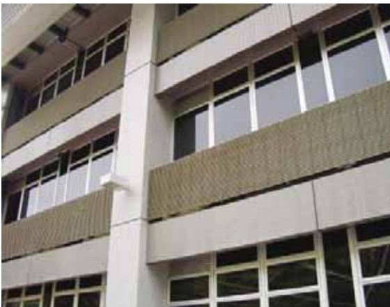
Above: DURADEK® pultruded fiberglass grating was installed as visually appealing louvers, concealing the air conditioning units of a school in Hong Kong.
