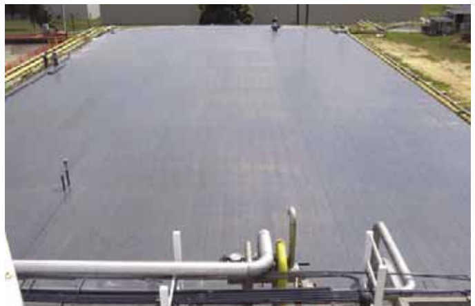
Above: An odor control cover was constructed using EXTREN® structural shapes for a waste water treatment facility in Puerto Rico. The second photo also shows the COMPOSOLITE® cover installed.
