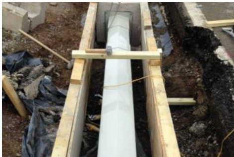
Linear PP-H drain former with timber shuttering to allow for concrete pour
