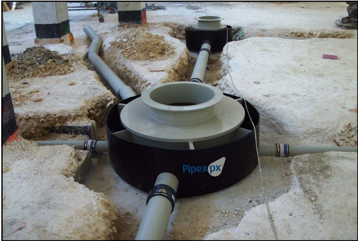
(Pipex px ® PP-H manhole during the installation process at Farsons Brewery, Malta)
